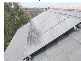
Bolt-on solar PV panels
